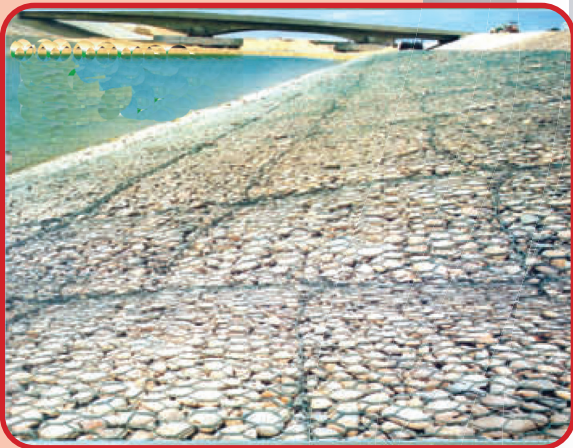
Gabions - Mattresses & Netting
